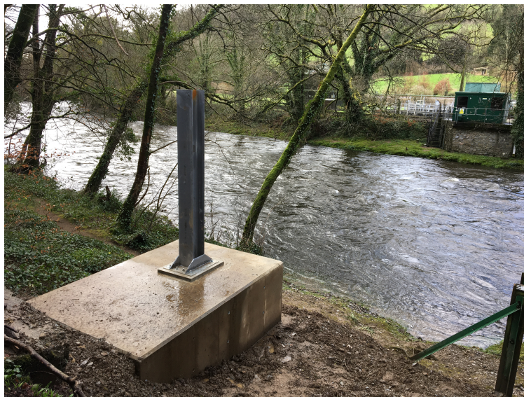
Figure 3: Image showing the presence of a new cableway stanchion installed in February 2020 (after the end of the field experiment documented here).
