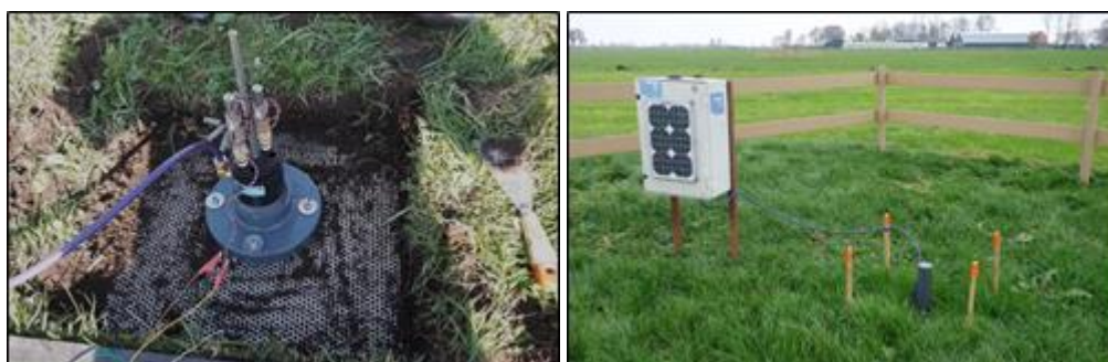
160 Figure 3. Left: extensometer head and stainless-steel plate a few centimetres below surface level. Right: extensometer protected by a PVC cover and connected to the datalogger with solar panels.
