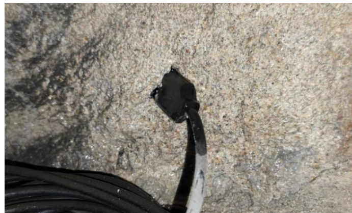
Figure S5. The installed FDR sensor in Cave #9.
