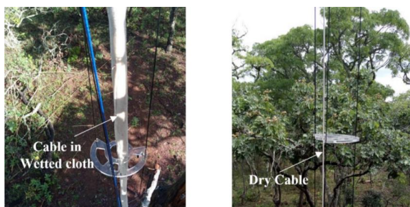
Figure 3. Installing the wet (left) and dry (right) fibre optic cable on the observation tower at Mpika site, Zambia. Under canopy view without screens.
