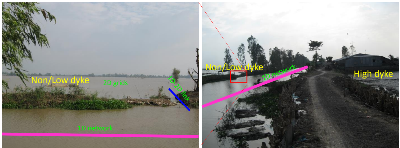
Figure 2. A high dyke and non/low dyke in An Giang province and their schematization in modelling. Photos by Vo Quoc Thanh 2012.
