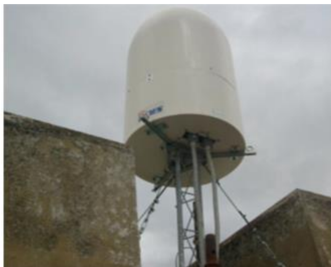
Fig. 3. WR-10X installation at Naples Castel Sant’Elmo site.
