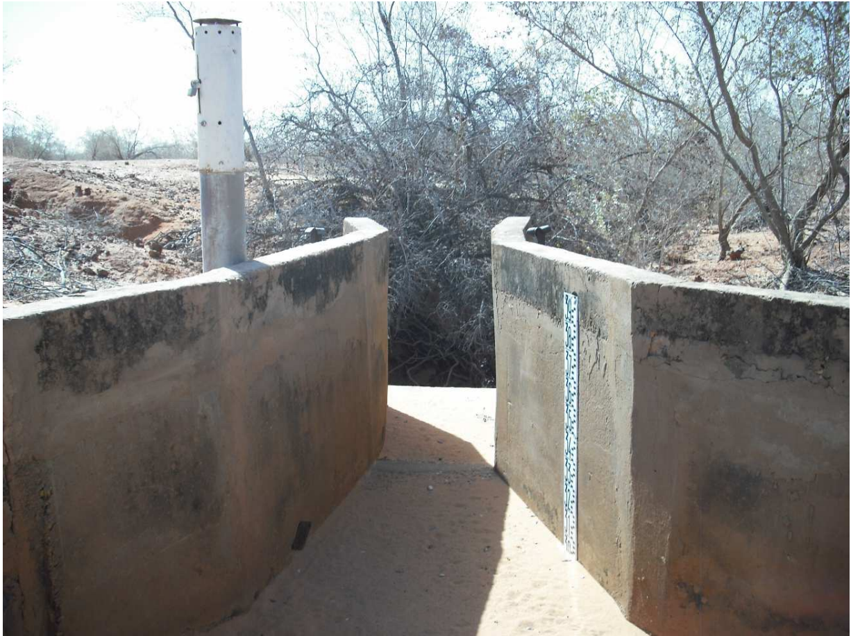
The streamgauge of the AMONT station
