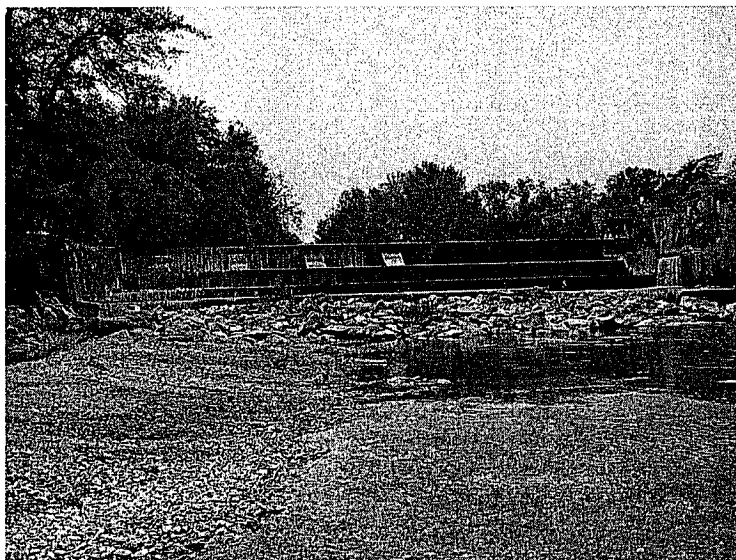
Fig. 4. River dam at low river discharge ( 9 \text{ m}^3/\text{s} ; 16 June 2006). Note, as evidence for the subsidence of the dam structure, that the crest is only overflowed on its left side (a diagram is given in Fig. 2).
