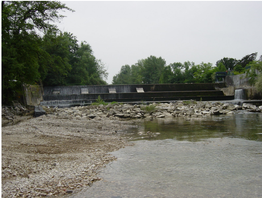
Fig. 4. River dam at low river discharge ( 9 \text{ m}^3/\text{s} ; 16 June 2006). Note, as evidence for the subsidence of the dam structure, that the crest is only overflowed on its left side (a diagram is given in Fig. 2).
