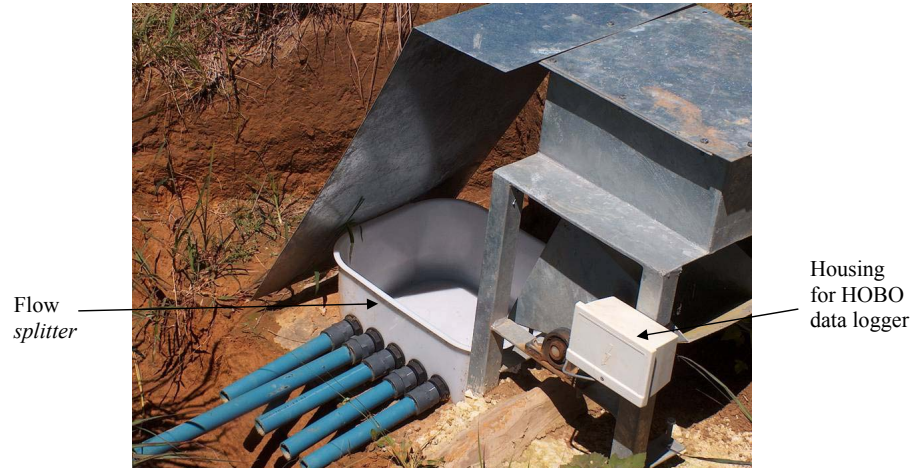
Fig. 7. A flow splitter attached to a tipping bucket, showing the five outlet pipes, only one of which drains to the sample tank.
