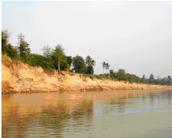
Fig. 10. Photographs showing streambank erosion along the Lower Mekong River in Vientiane, Laos.
