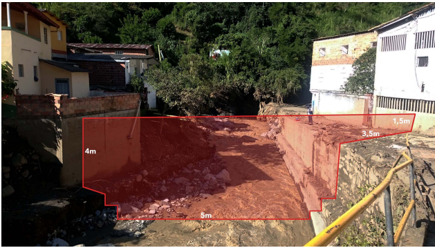
Figure 4. Channel cross section showing an example of flooded infrastructure during the flash flood event. The section shows mud marks on the walls of adjacent houses, with heights varying between 0.5 and 1.2 m. The houses in the picture are located 4–5 m away from the channel. The photograph also shows the width of the channel and the total estimated depth during the flash flood. The cross section is downstream from the bridge shown in the picture.
